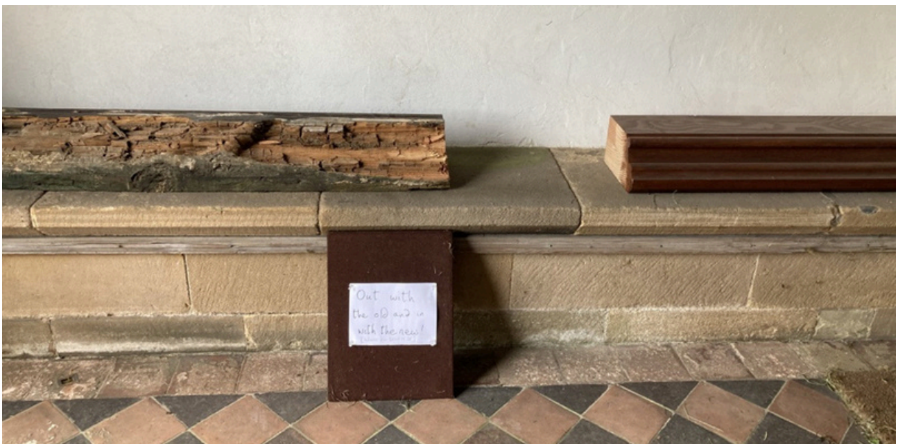
Dry rot and its replacement 2025. Photo: Richard Bimson.
