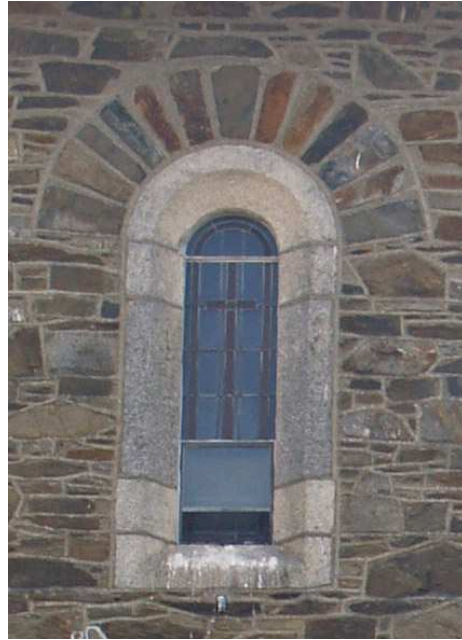
Pugin's sketch for the builder, Richard Pierce, illustrating stone arrangement for windows (left) (Source: Forde, pp. 76–7) and a typical clerestory window as constructed (right) (Image: Brian Andrews)
